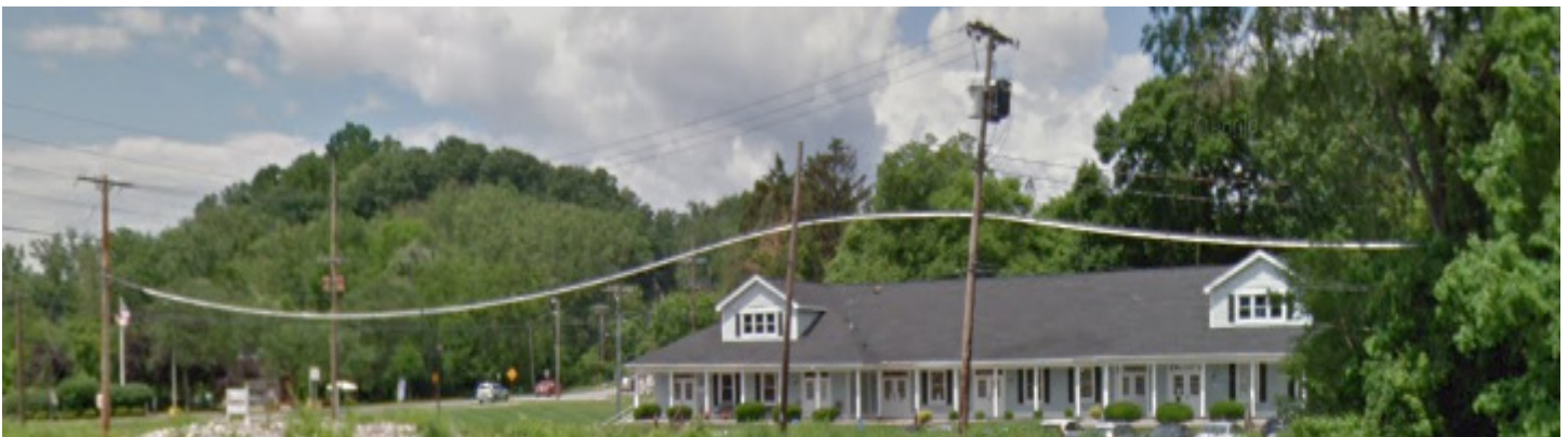
Circuit 759 at Penfield Road: A Nitrogen-Filled Electric Aerial Cable.
