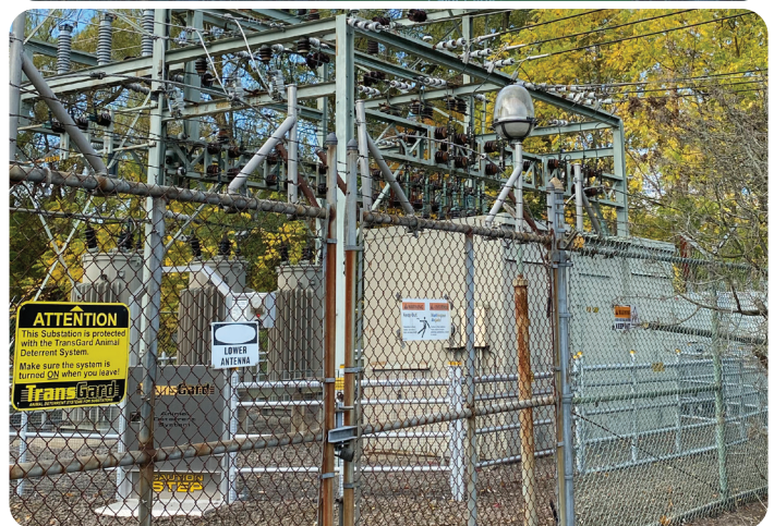
As part of the upgrade, a new substation will be built on the acquired adjacent parcel and the equipment at the existing substation will be removed (center and bottom images). Having exceeded its peak load capacity in the past, the infrastructure upgrade to Substation 192 will include replacing the existing transformer with a new, more efficient model to support its three existing distribution circuits. The enhanced capacity will provide critical redundancy contingencies for adjacent circuits that are currently without adequate circuit reinforcements during high demand periods.
