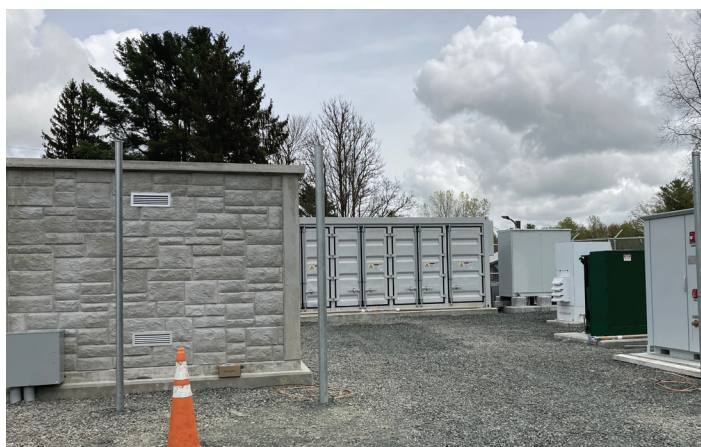
BESS Site Entrance
