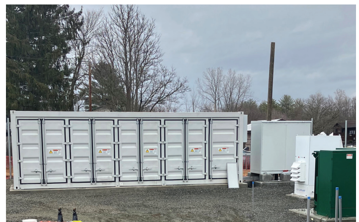
BESS Site Interior
