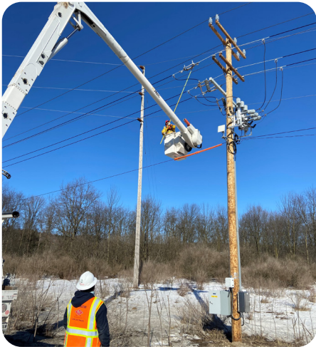
The Langner Road substation project installed state-of-the-art equipment, including 25 smart circuit devices, to help increase reliability for our customers.
